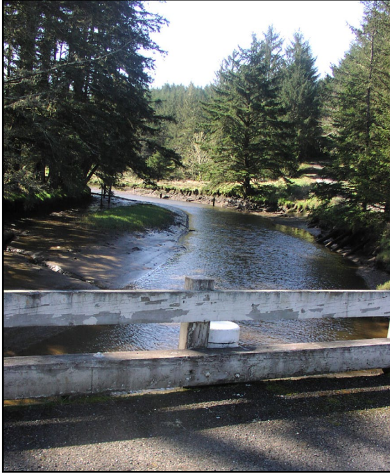
Figure 7.3: Hinch Bridge, located in the relatively remote southern end of the Reserve, is a hot-spot for vandalism. This is in part due to its accessibility.
