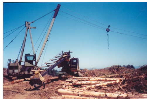
Figure 2.14: A yarder, which uses a system of cables to pull felled logs up to the landing where they can be processed for transport.
